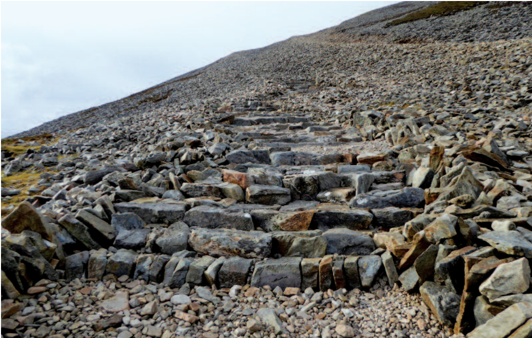
View of the 40-metre pilot path work on the lower part of Croagh Patrick's summit cone; the technique used provides a stable path that fits into the landscape.
